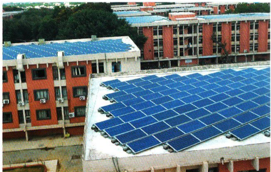
Hartek Solar's rooftop solar installations in Chandigarh locality
